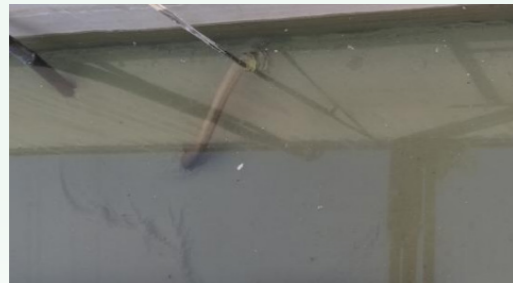
Sludge pump of raw water tank
