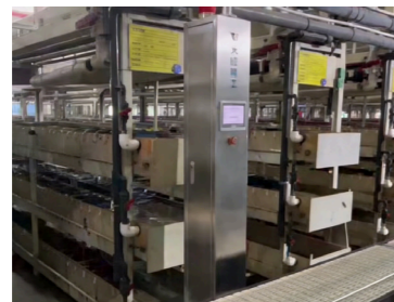
Intelligent Inspection Robot
