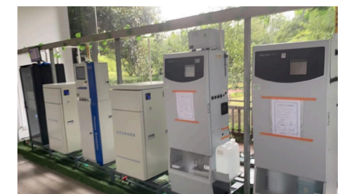
Online Automatic Monitoring Facility of Pollutant Source
