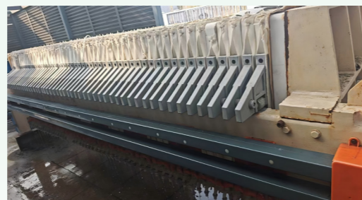
Sludge filter press device
