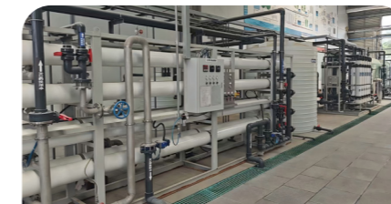
Reverse osmosis equipment for reclaimed water reuse
