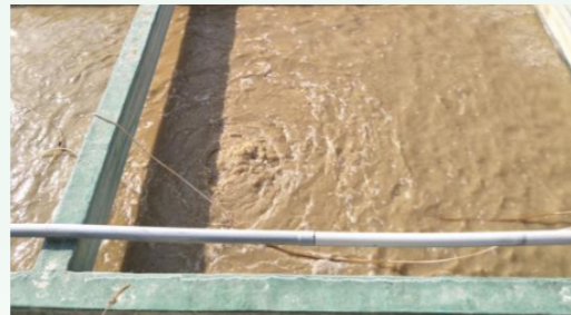
Aeration in sludge tank
