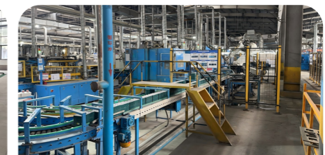
Reclaimed water and circulating water are reused in the workshop for production
