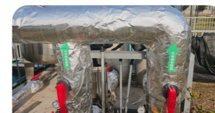
Additional recovery pipe network and water pump in the plant
